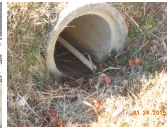
Irrigation Pipe thru Culvert
